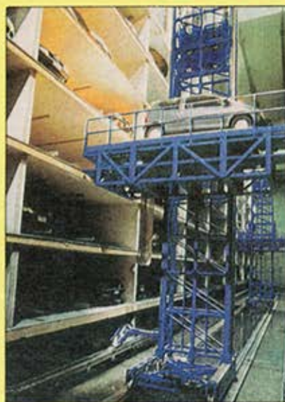
INTELLIGENT AUTOMATIC MECHANICAL CAR PARKING
