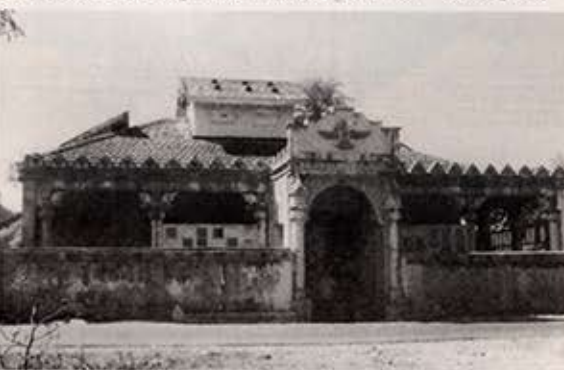
N. F. Goiporia Dar-e-Meher at Davier: in need of repair
