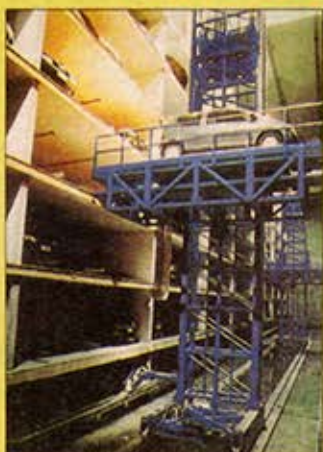
INTELLIGENT AUTOMATIC MECHANICAL CAR PARKING
