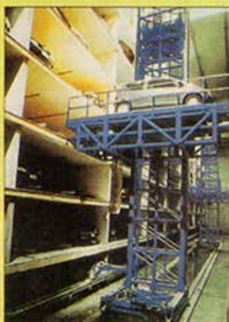
INTELLIGENT AUTOMATIC MECHANICAL CAR PARKING
