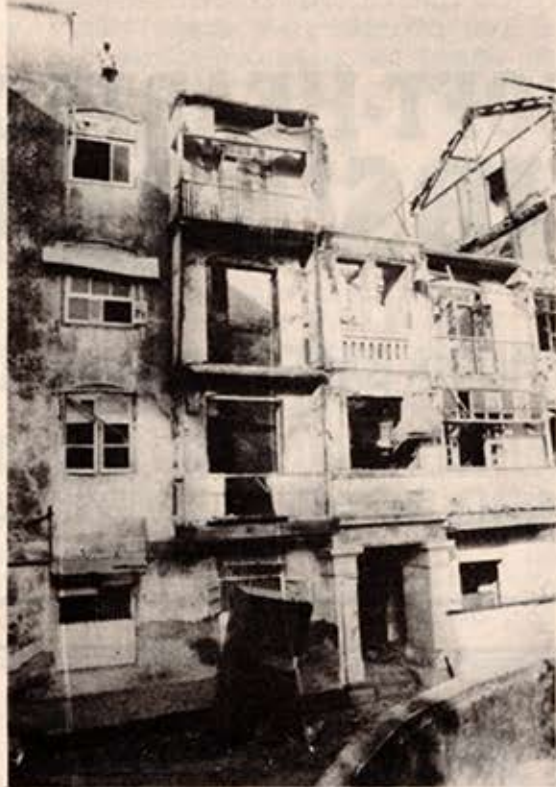
The gutted G block at Dalal Estate
