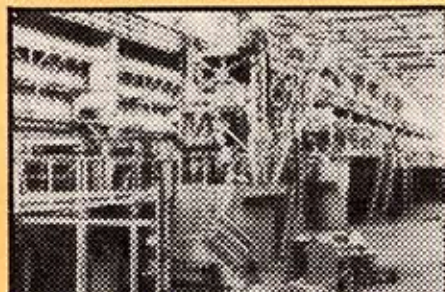
Salem Steel Plant: Annealing and pickling lines for stainless steel strip
