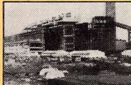
Visakhapatnam Steel Project: Thermal power plant and blower house with three 60 MW turbo-generator units
