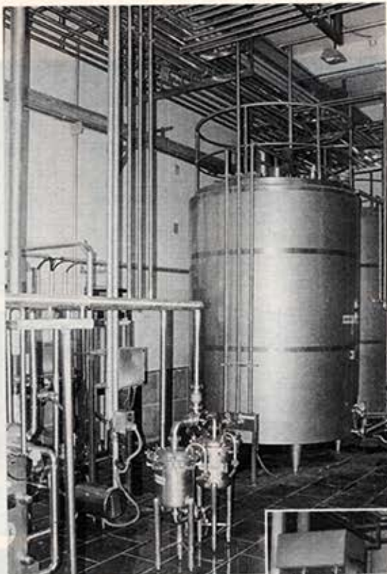
At the ice cream factory: mix preparation (left) and automatic bulk filling line
